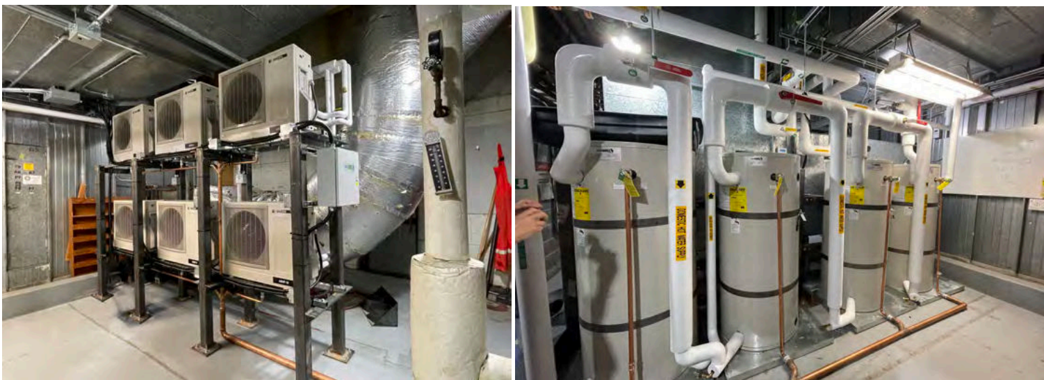
Installed system shown with 6 x Heat Pumps, 4 x SAN-119 gallon tanks and the SANCO 2 Controller for the system
